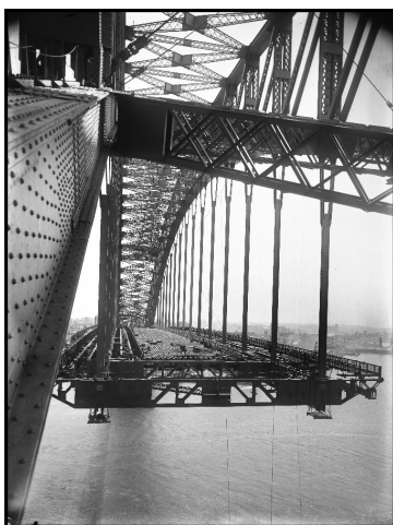
Sydney Harbour Bridge – decking from a cross lateral, Thursday 11 th Dec 1930. Photography by Rev. Frank Cash
