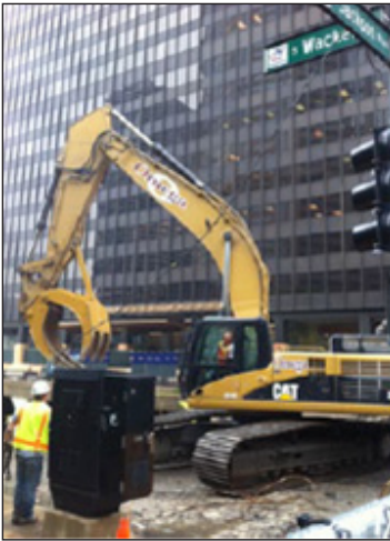
Construction continues in front of ATLA Headquarters on South Wacker Drive in Chicago.
